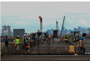
Construction work continues at a site in Caloocan City on December 6, 2022. STAR / Jesse Bustos
